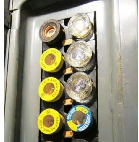
Typical screw-in fuse panel.
